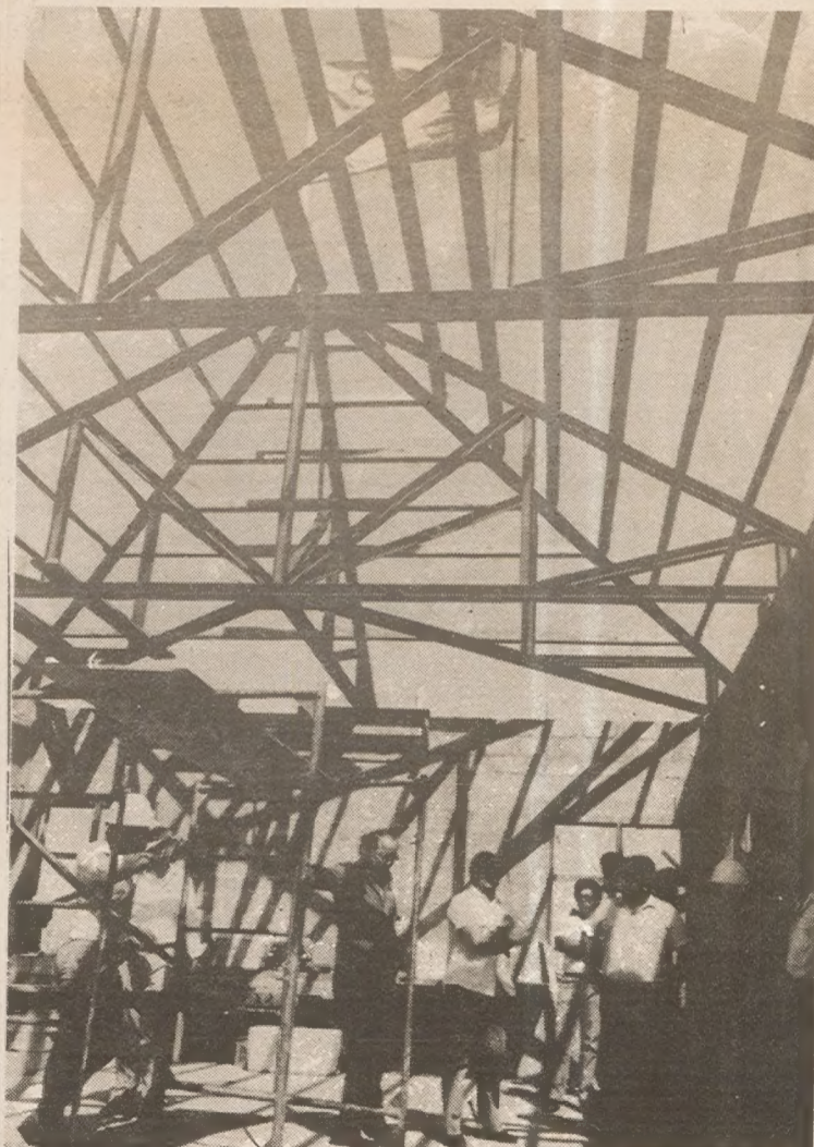
ORANJESTAD — The flag was raised on the rafters of the Public Works expansion project Friday afternoon and the traditional beer was drunk. The new building will house the building and Housing control office on the ground floor and the Civil Designs office will be on the top floor. Contractor Dijkhoff is the building contractor. The project which is scheduled to be finished in December, represents an investment of Naf.500,000.
